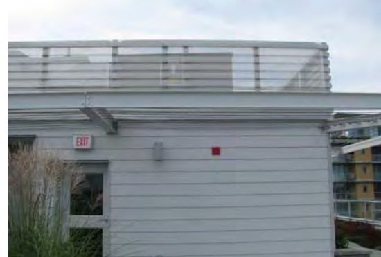
Architectural screening of rooftop mechanical equipment.
